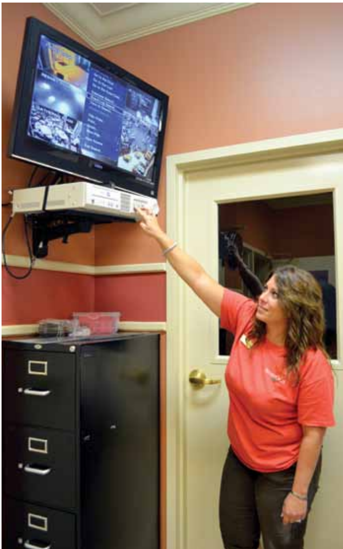
Theresa Flores, Clubhouse Manager, can view all 16 cameras simultaneous on this monitor. She can also view the parking lot and slide cameras on a second monitor in her office.
